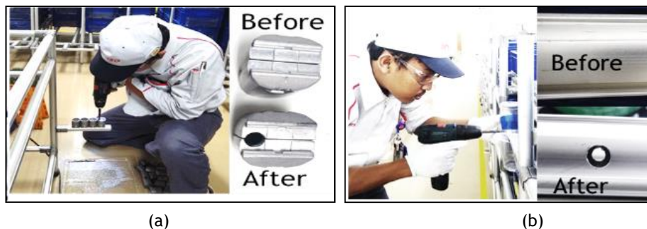
Figure 16. The installation of LED indicators; (a) drilling a connecting bar; (b) drilling the middle point below a drawer.
