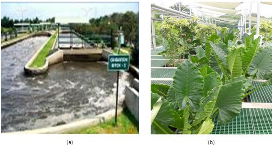
Fig 2. Appearance of WWTP using conventional oxidation ditch (a) and WWTP after with Organica-FCR technology (b) source: Documentation of Jababeka
