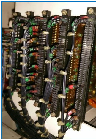
Gambar 6. Main Board Master Controller
